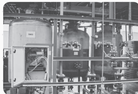
Control of pressure operated valves in battery recycling unit
